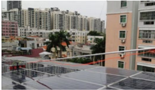
Solar panel system
